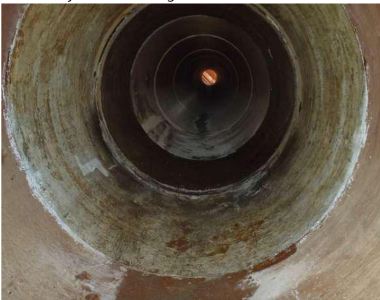
Location of deteriorated gasket
