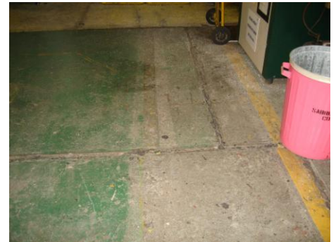
Before: Aging concrete floor
