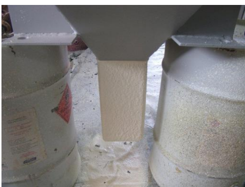
External coating of ore chute
